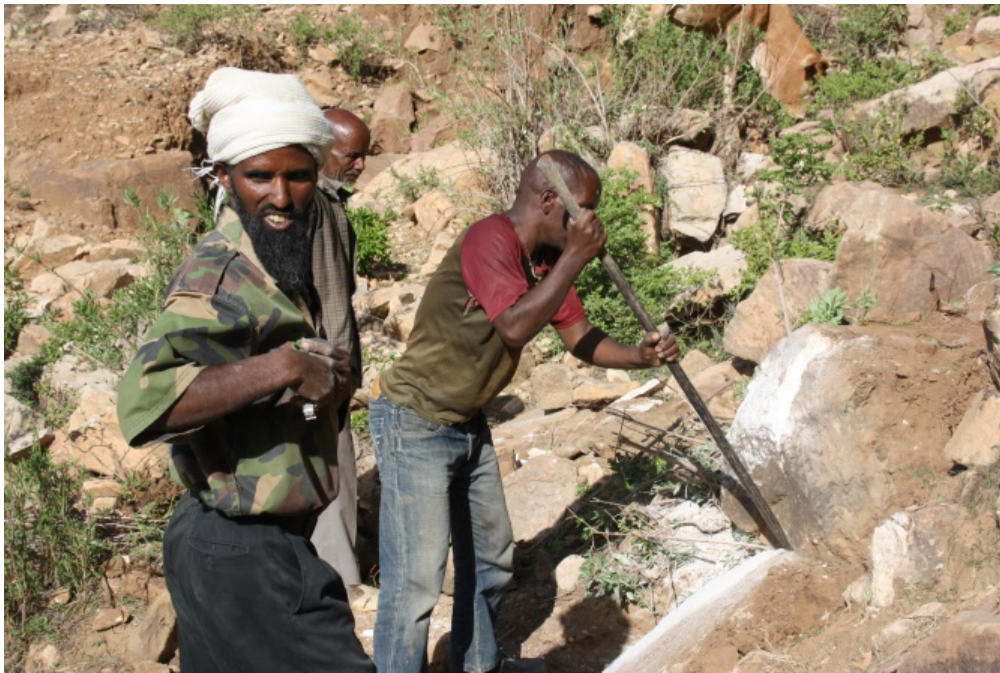
Figure 6. Men applying leverage with a pry bar to extract the boulder during excavation.
