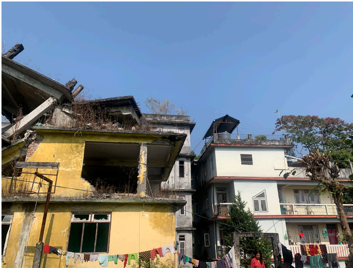
Figure 3: Broken houses tilting over neighboring buildings.
