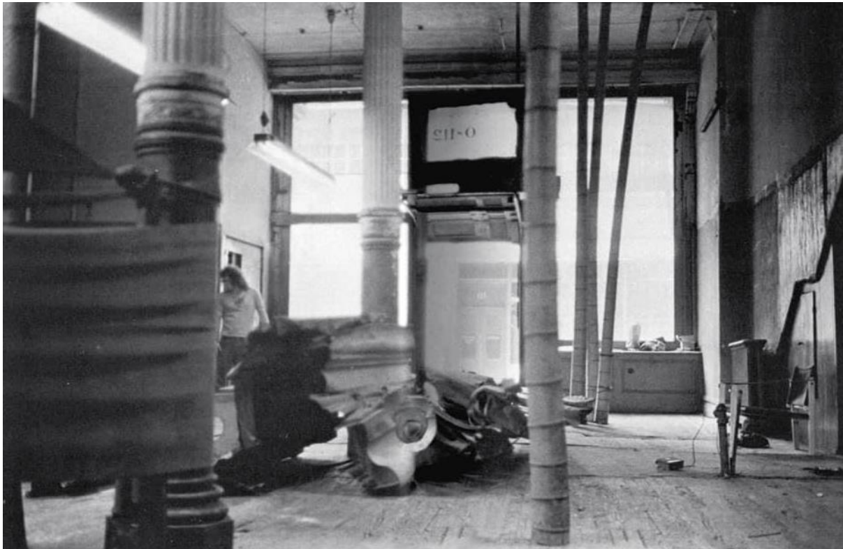
Figure 1: Installation in progress at 112 Greene Street, 1970 (Photograph by Alan Saret. In Alternative Art New York, 1965-1985 , edited by Julie Ault. Minneapolis, MN: University of Minnesota Press, 2002, 255).
